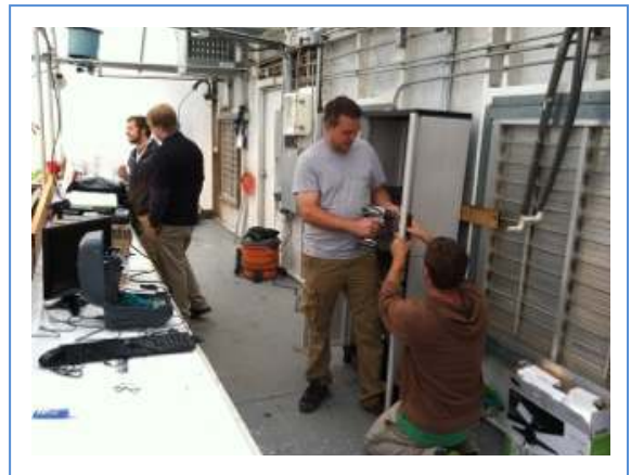
Installing system in a protected cabinet at the back of the greenhouse
